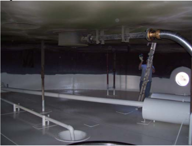
A new coat of paint on the inside. The roof “floats” above the fuel and is seen at the top of the picture above.
