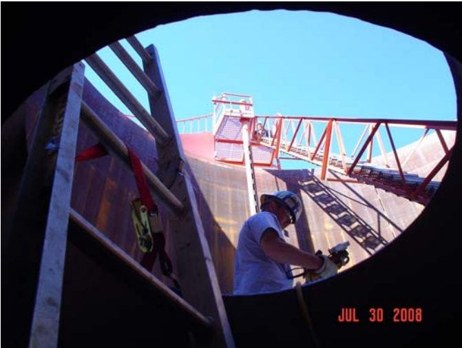
A shot of the open hatch in the roof to allow access.
