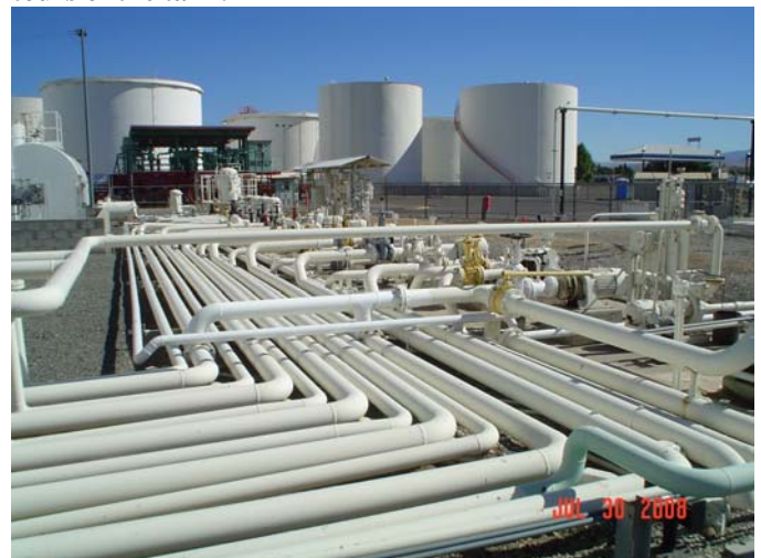
Piping from the tanks to the loading racks
